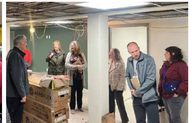
Currently under construction, Wayne County's walk-in Crisis/Stabilization Center will provide immediate mental health care services including medication management and short-term residential support.
