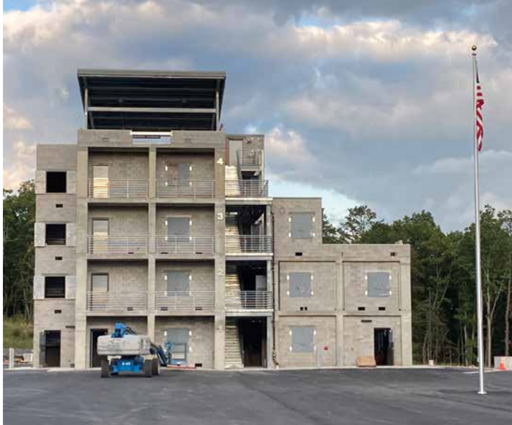
The four-story fire training tower will serve as the focal point for high angle rescue and fire suppression exercises.
